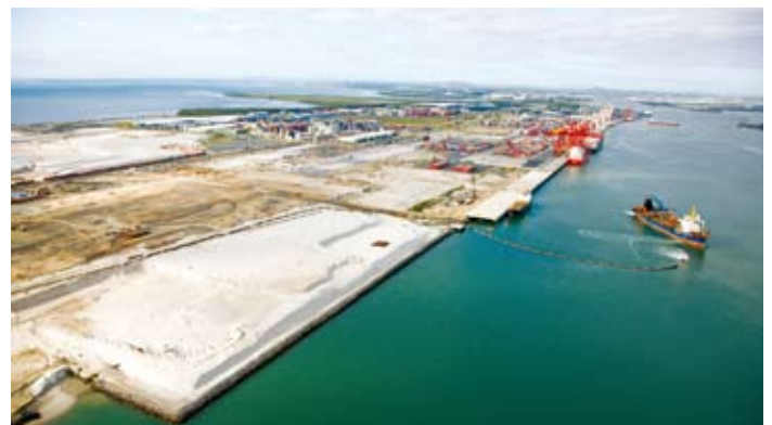
Sand surcharge placement, behind the recently completed Berth 11 rockwall and up to the Terminal 11 trial area, is almost complete.
